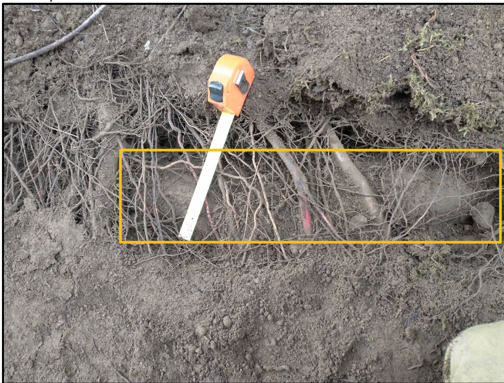
Photograph 6. Largest root encountered on site. Root measured 4.5 inches and grows horizontally along trench. Root should be preserved and excavation should not occur within 16 feet of the trunk of Tree 13.
