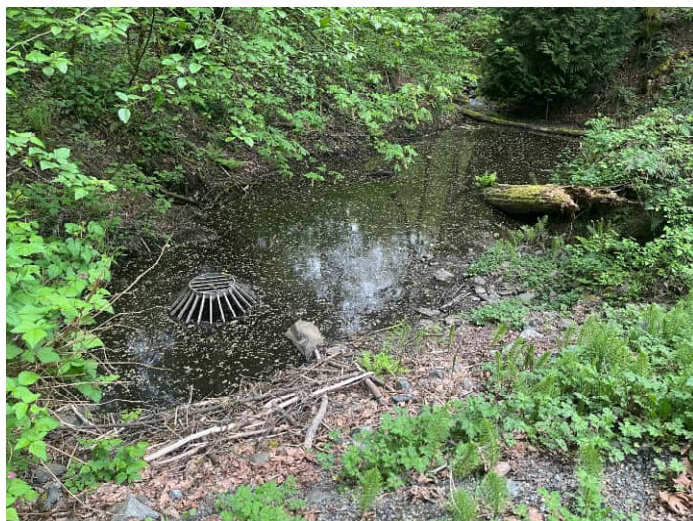
A view of the sediment pond at E Mercer Way, facing upstream.
