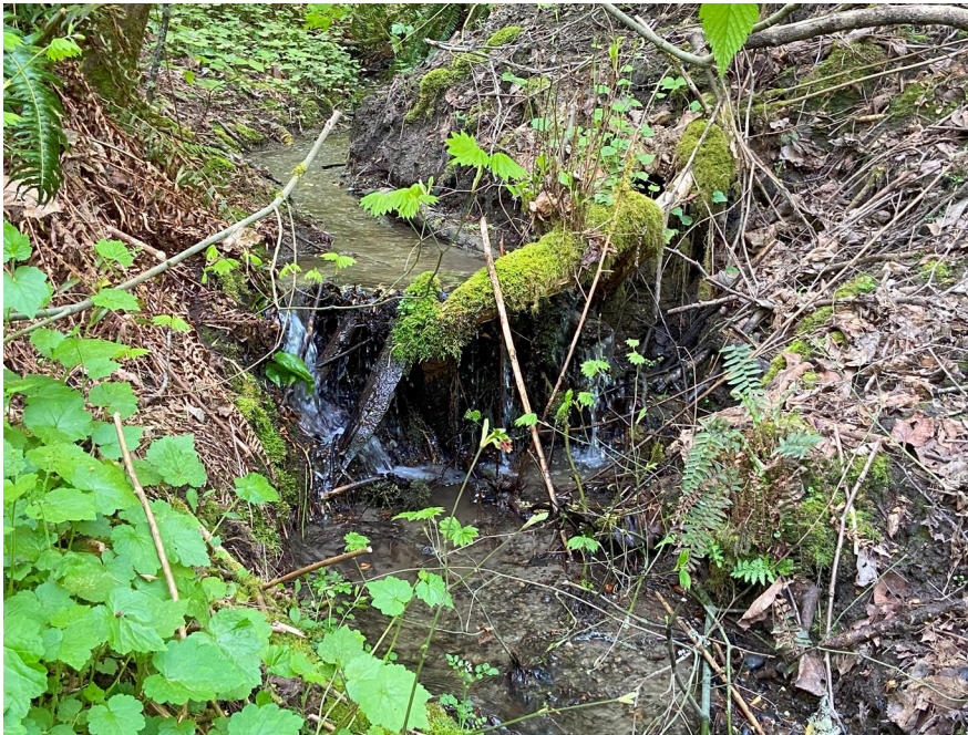
Photo 2.2 Upstream view of stream channel, about 560 feet upstream of EMW. Note, existing debris in channel providing limited grade control and some upstream sediment retention and flanking with erosion along channel banks.
